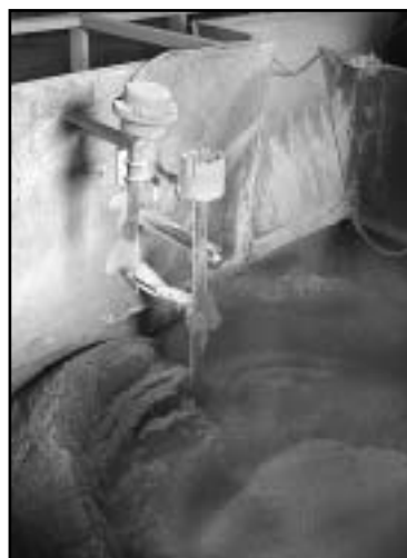
A concrete manufacturing plant has installed a new Model KA unit in the pictured bin. This bin is filled with stone, but Model KAs are also being used in this facility with steamed sand, gravel and cement.
