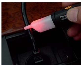
Incorrect phase sequence
